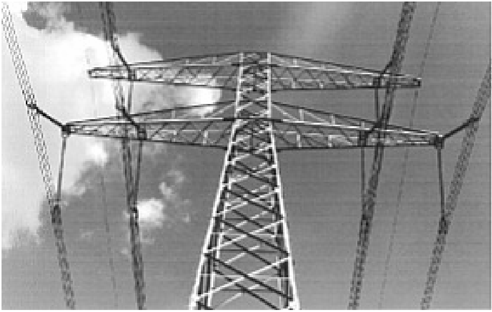
Transmission line tower
